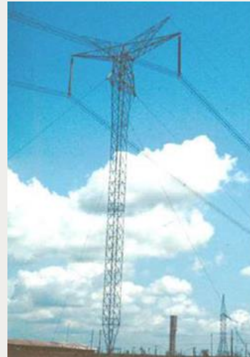
TL +/- 600 kV – Foz de Iguaçu – Ibiúna
